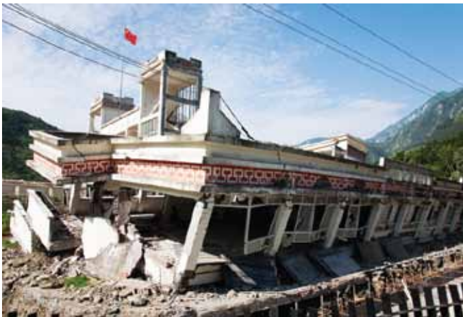
A school collapsed during the Sichuan Wenchuan earthquake 在汶川地震中倒塌的校舍
